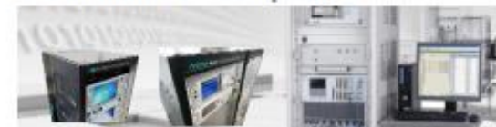
Data Center / Computing
